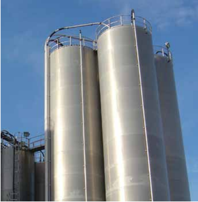
| Total Petrochemicals monitors energy use in its production process
